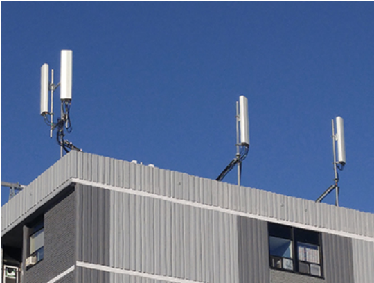
Figure 2: Directional antennae on the roof of a building.
