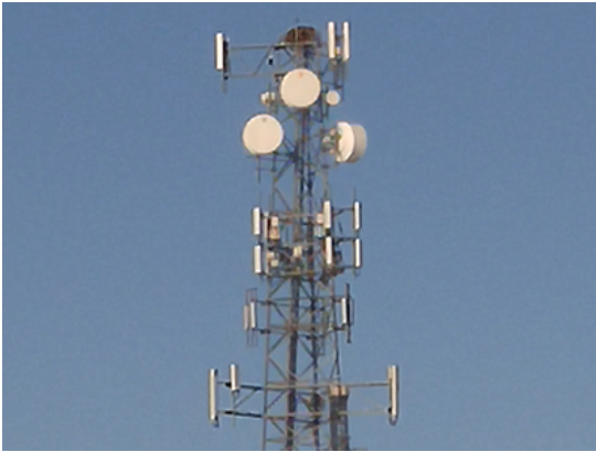
Figure 1: Directional antennae on a tower.
